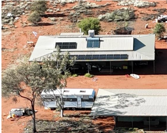
New Solar Panels and 300l Solarhart HWS
