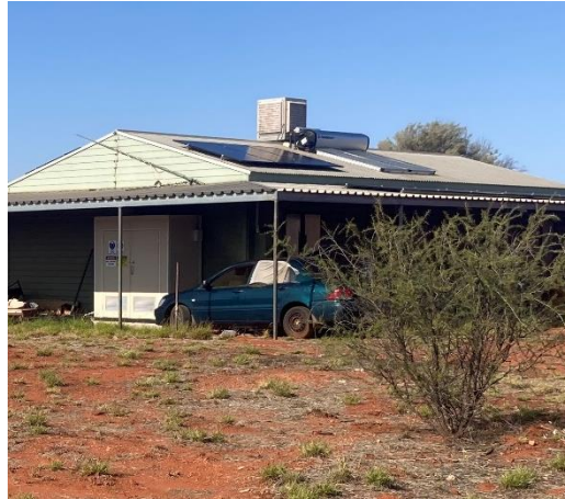
New Solar Panels and 300l Solarhart HWS
