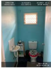
Toilet. Replacement of sink and toilet bowl supply and install grab rails for support AS per standards to suit Tenans's needs
