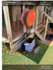
fire hose reel Replacement of the existing fire hose reel as its old, damaged and short it doesn't reach everywhere around the house incase of fire.
