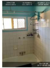
Bathroom remodel Complete demolition of the bathroom removal of all thab, vanity, tiles, Wall lining and painting
