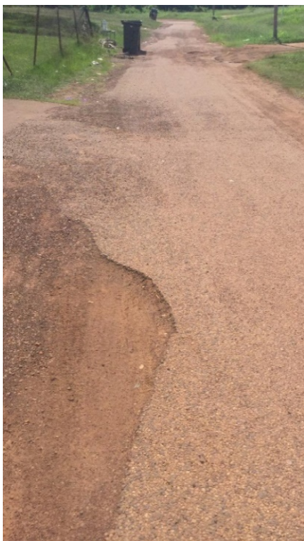
Figure 10 Typical sealed road, condition: poor
