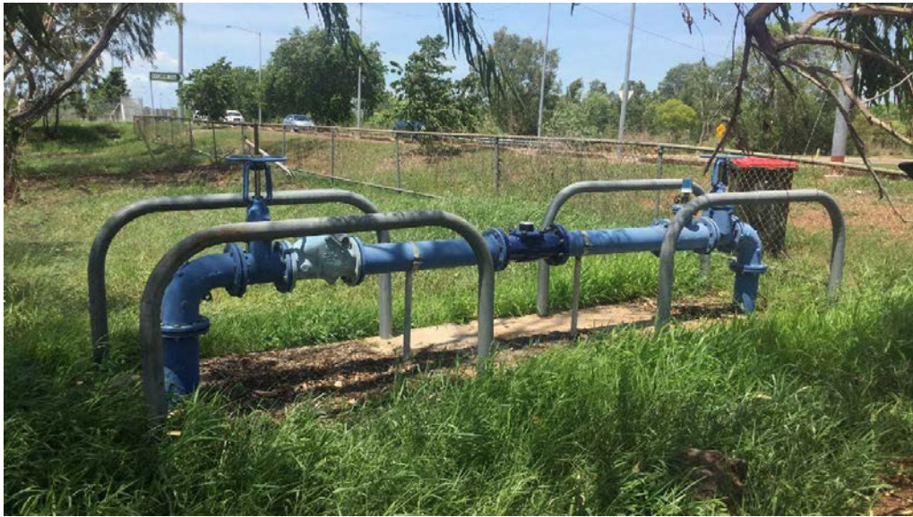
Figure 5 Water meter (bulk), condition: very good
