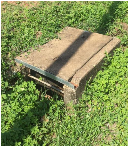
Figure 9 Letterbox pit, condition: good
