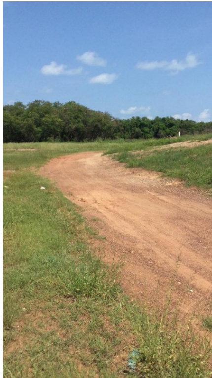
Figure 11 Typical unsealed road, condition: poor
