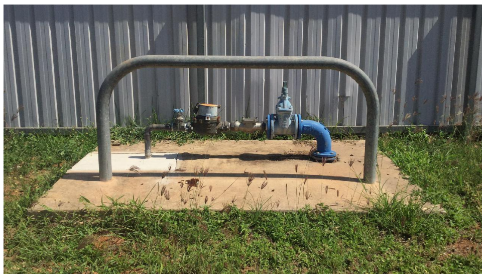
Figure 3 Water meter (bulk), condition: good
