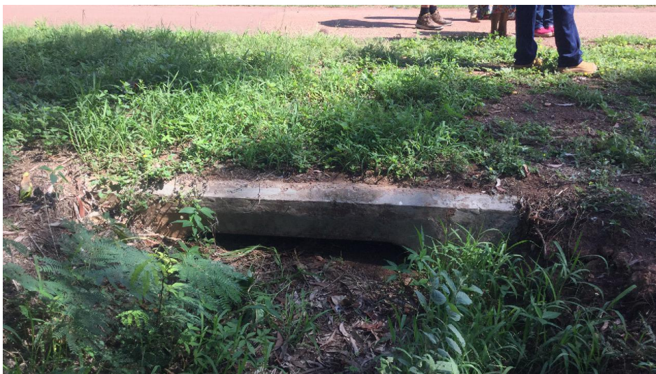
Figure 8 Culvert, condition: poor
