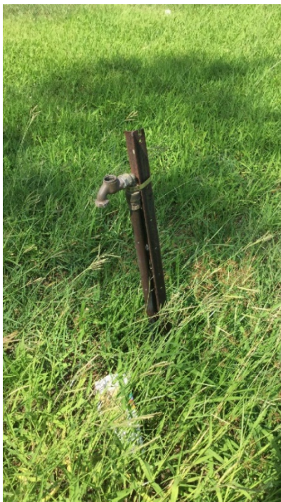
Figure 6 Tap, condition: very poor
