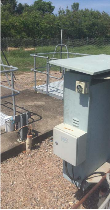
Figure 1 Pump station, condition: good
