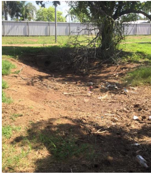
Figure 10 Swale, condition: poor
