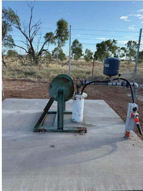
Roller installed control panel to be install
