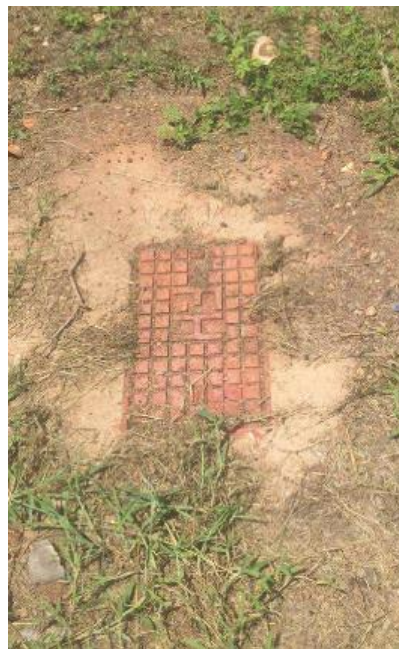
Figure 6 Fire hydrant, condition: poor
