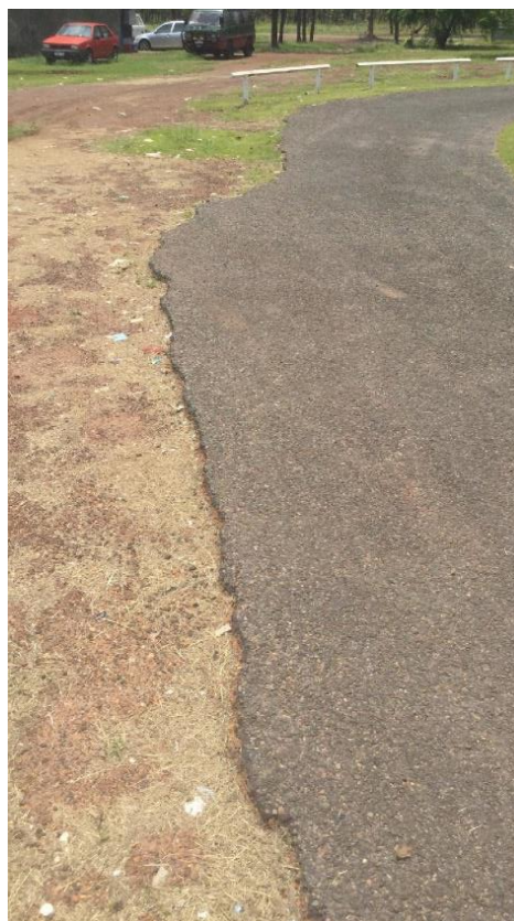
Figure 8 Pavement edge breaks, condition: poor
