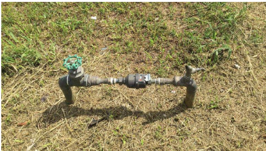
Figure 6 Water meter (lot), condition: good
