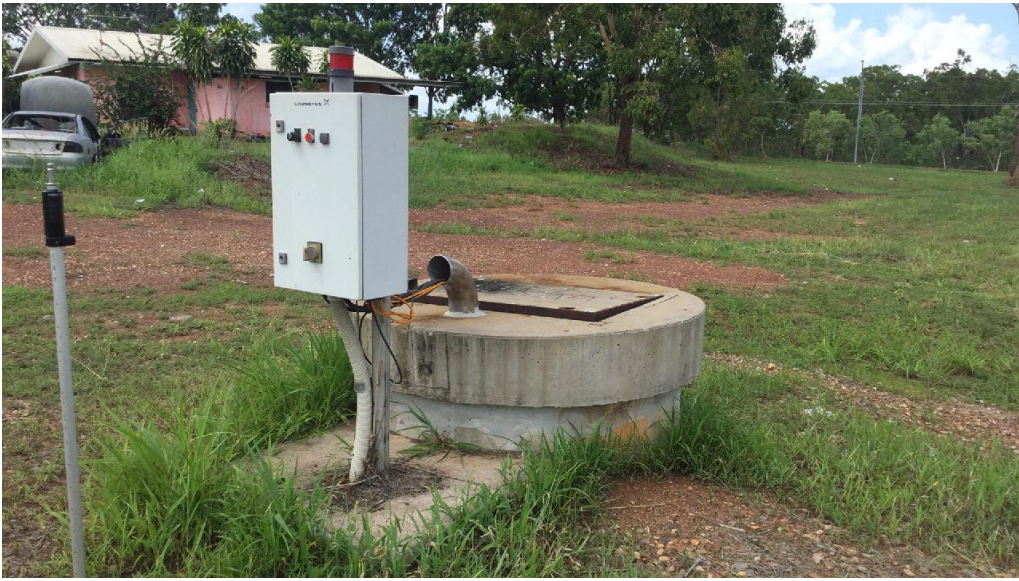
Figure 1 Temporary sewage pump station at Palmerston Town Camp
