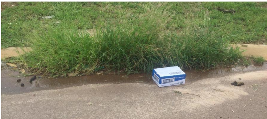
Figure 11 Side entry pit, condition: good (structure good, blockage very poor)
