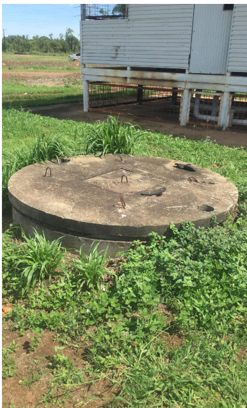
Figure 1 Septic tank outside ablution block
