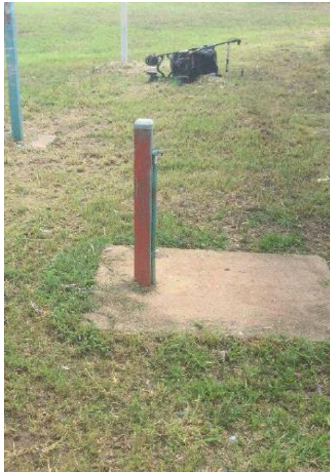
Figure 5 Tap, condition: very poor
