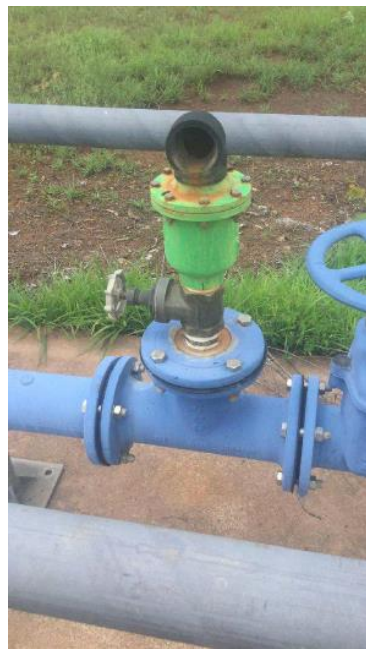
Figure 5 Air valve, condition: good
