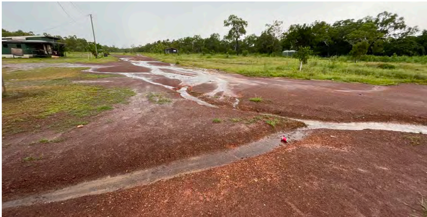
Before photo of stormwater damage to internal road and main intersection, view towards east
