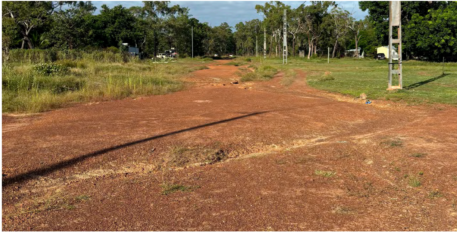
Before photo of stormwater damage to the internal road running north/ south
