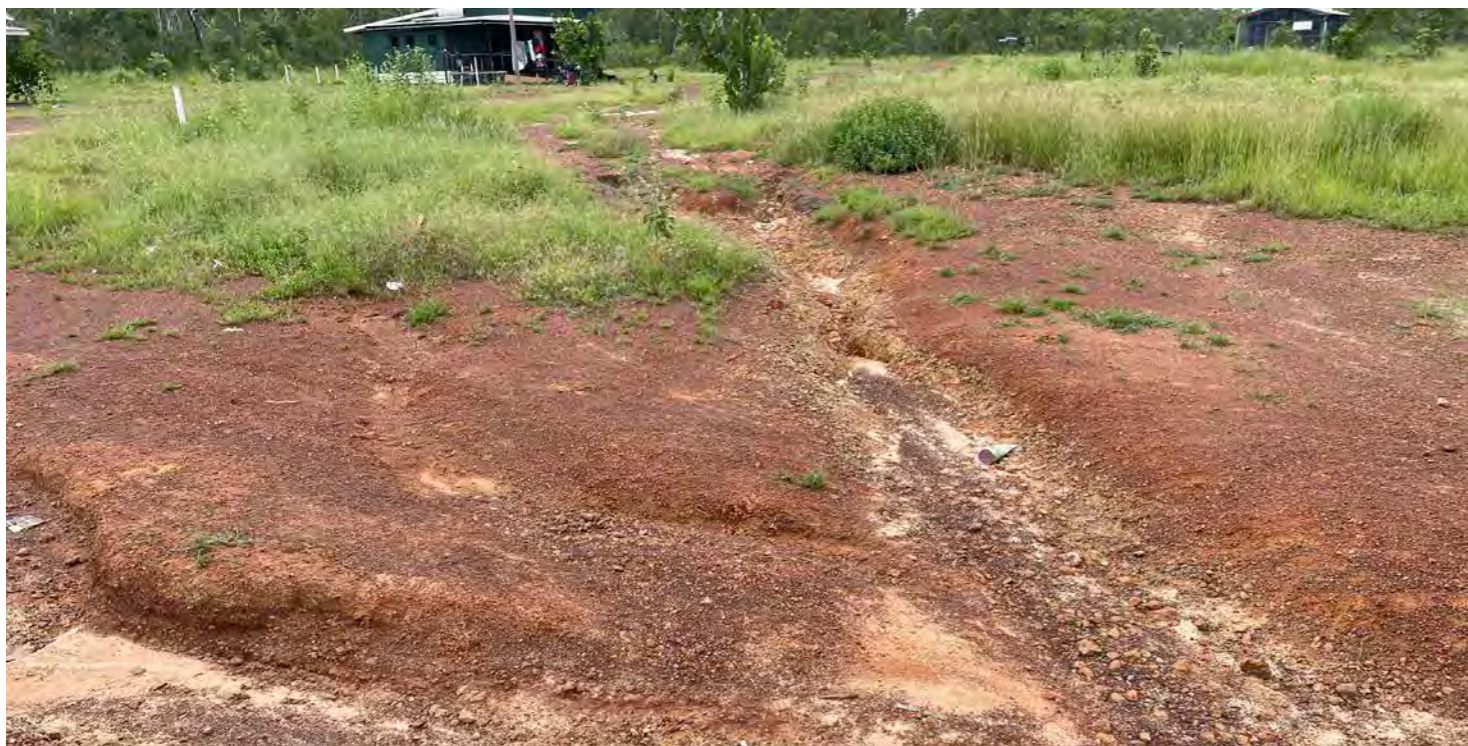
Before photo of stormwater damage to internal road, view towards east
