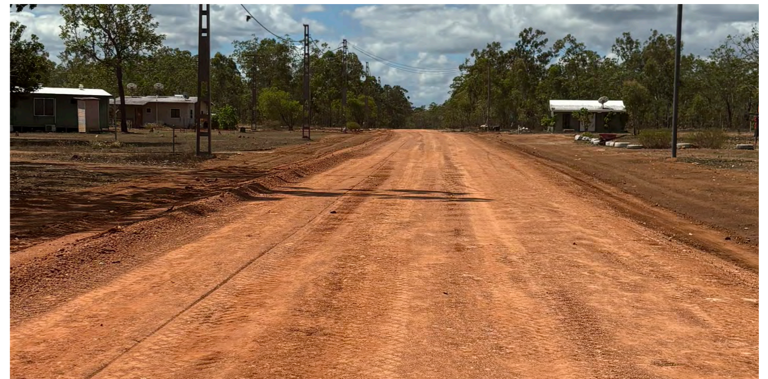
Photo of internal road works in progress, internal road running east/ west
