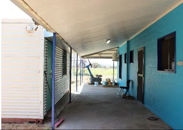
Veranda Ceiling to Sleepout area and box gutter:
