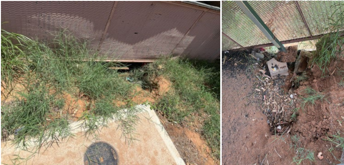
Figure 62. Eroded backfill around septic tank
