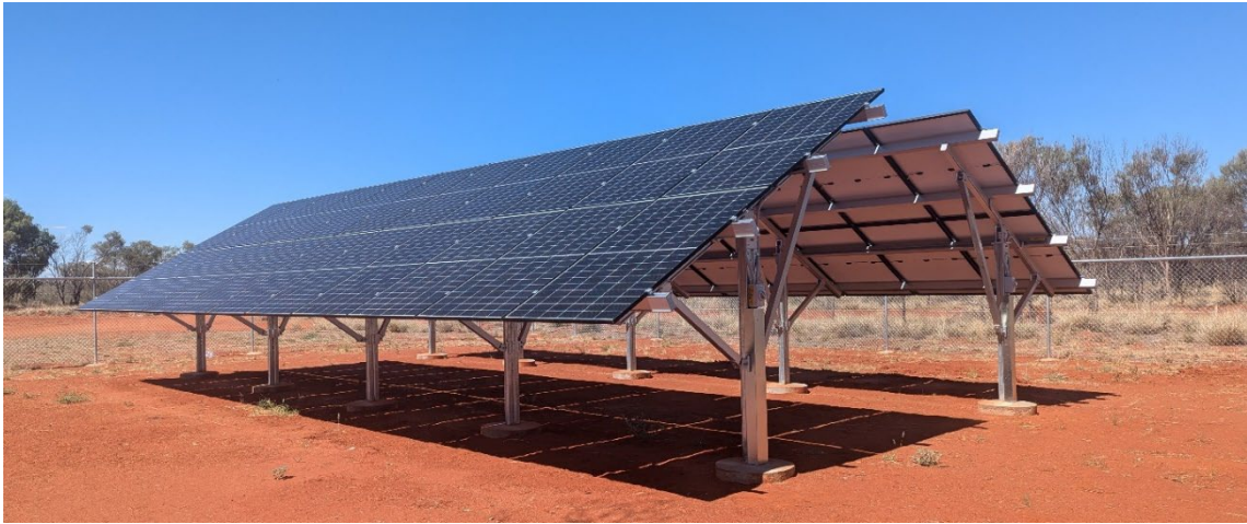
Figure 46. New solar array at Burt Creek
