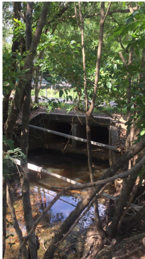
Figure 11 Culverts and drain with ponding
