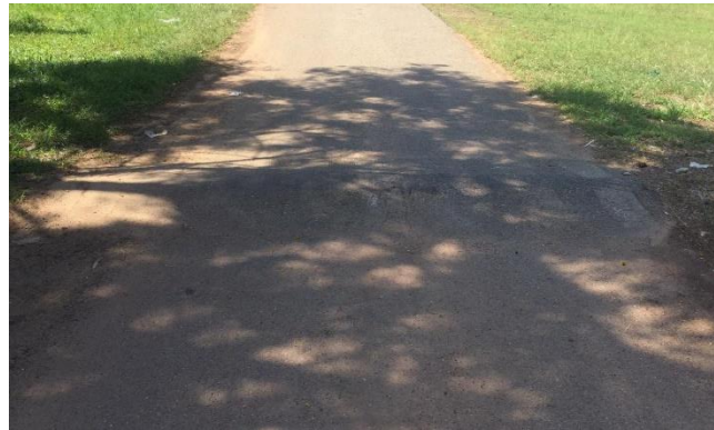
Figure 8 Speed hump, condition: poor
