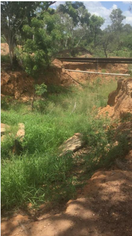
Figure 7 Swale, condition: very poor
