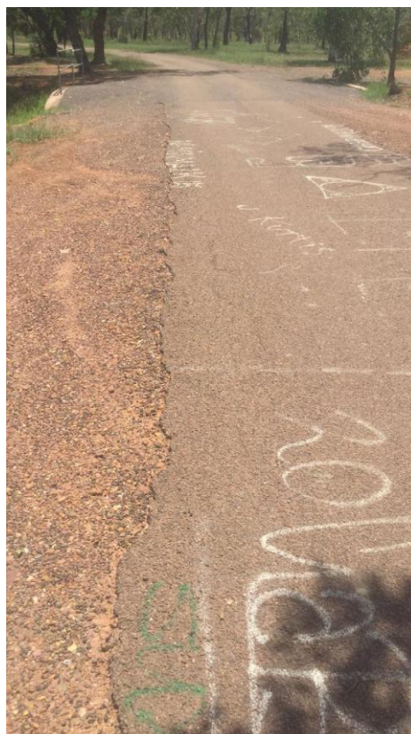
Figure 6 Pavement, condition: poor
