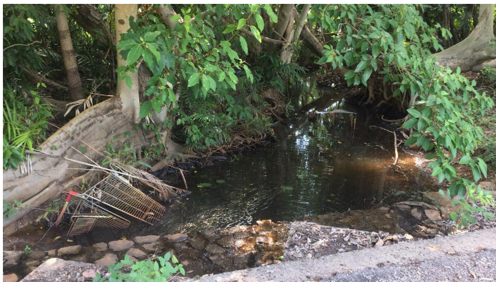
Figure 12 Drain with ponding and debris at Railway Dam
