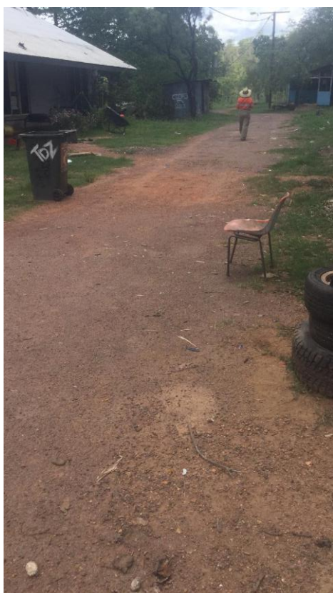
Figure 5 Pavement, condition: very poor
