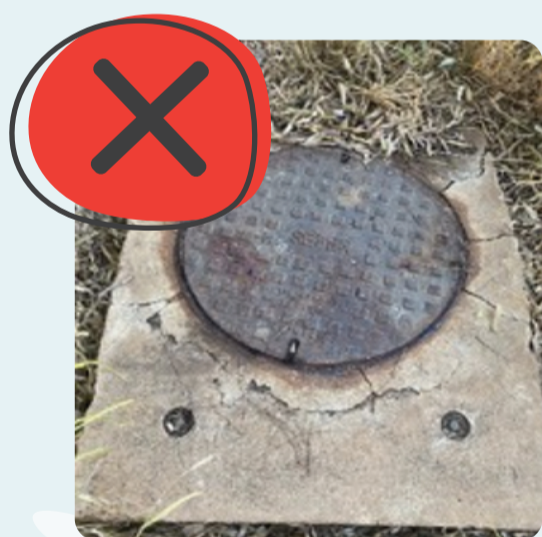
Cracked lid or concrete
