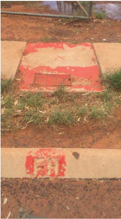
Figure 5 Fire hydrant, condition: poor
