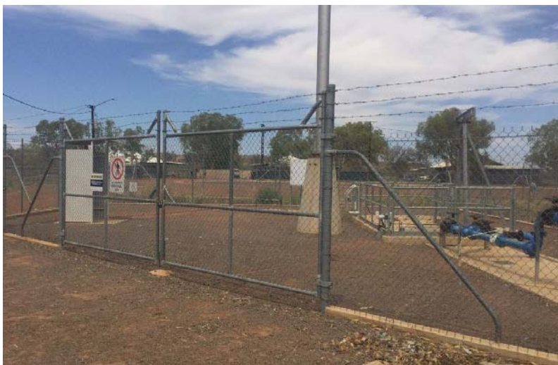
Figure 3 Sewage pump station, condition: good
