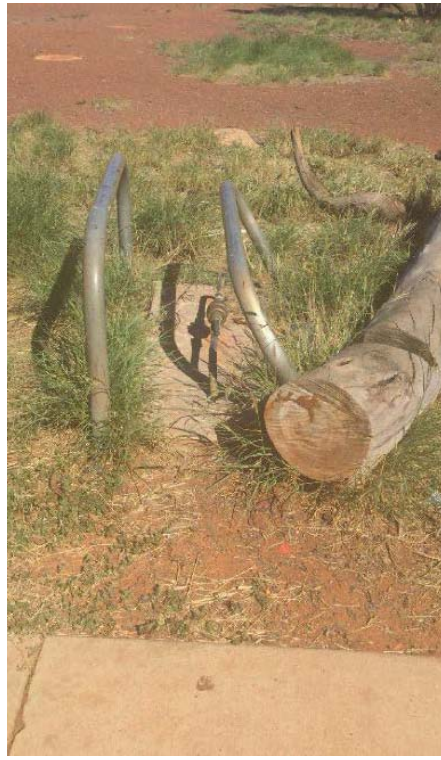
Figure 6 Water meter (residential lot), condition: poor
