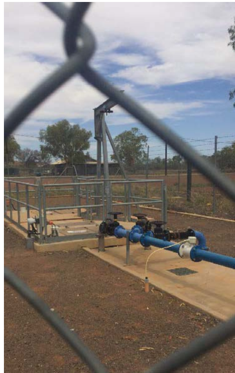
Figure 2 Sewage pump station, condition: good
