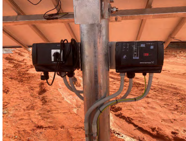
Bore pump controller:
