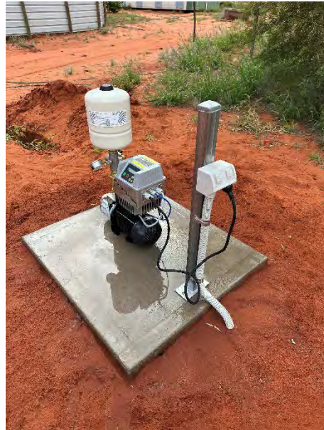
New pressure pump:
