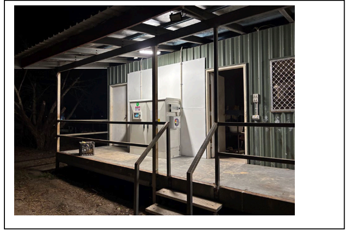
New inverter enclosure
