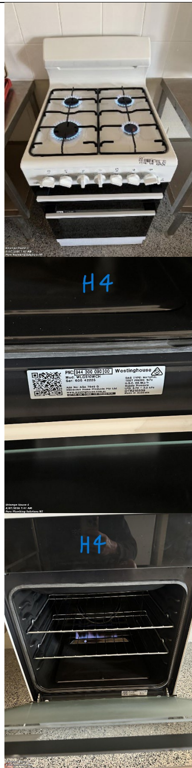
New LPG Gas Cooker installed 08.07.2026. Gas Compliance # 446618
