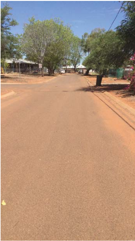
Figure 8 Wilyugu Street, condition: good
