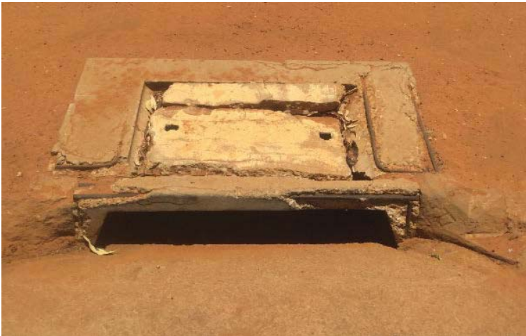
Figure 12 One bay side entry pit, condition: poor
