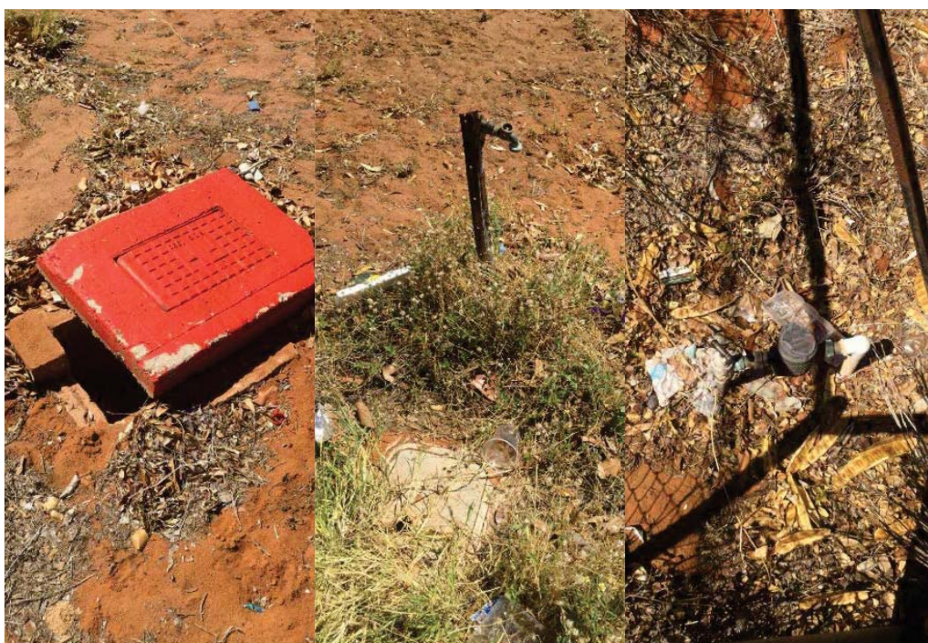
Figure 2 Fire hydrant, condition: very poor
