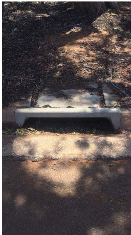
Figure 11 One bay side entry pit, condition: poor
