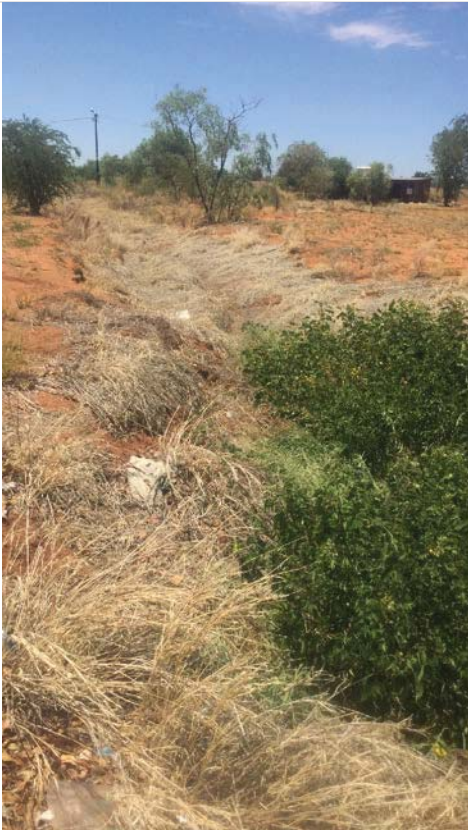
Figure 10 Swale, condition: poor
