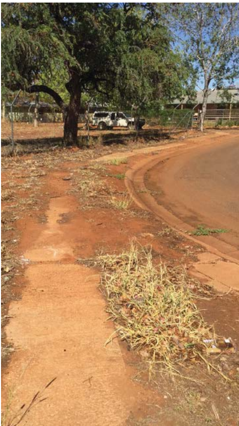
Figure 5 Footpath, condition: poor
