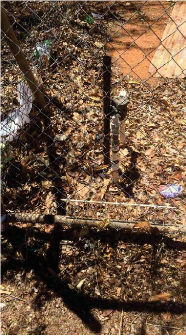
Figure 4 Water meter (lot), condition: poor
