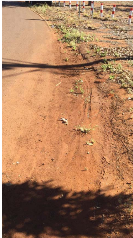
Figure 9 Ijibarda Street, gutters filled with dirt, condition: poor
