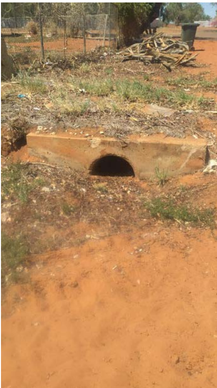
Figure 10 Culvert endwall, condition: good , blockage: 50%
