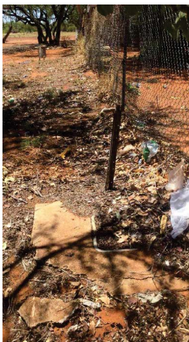
Figure 3 Tap, condition: very poor
