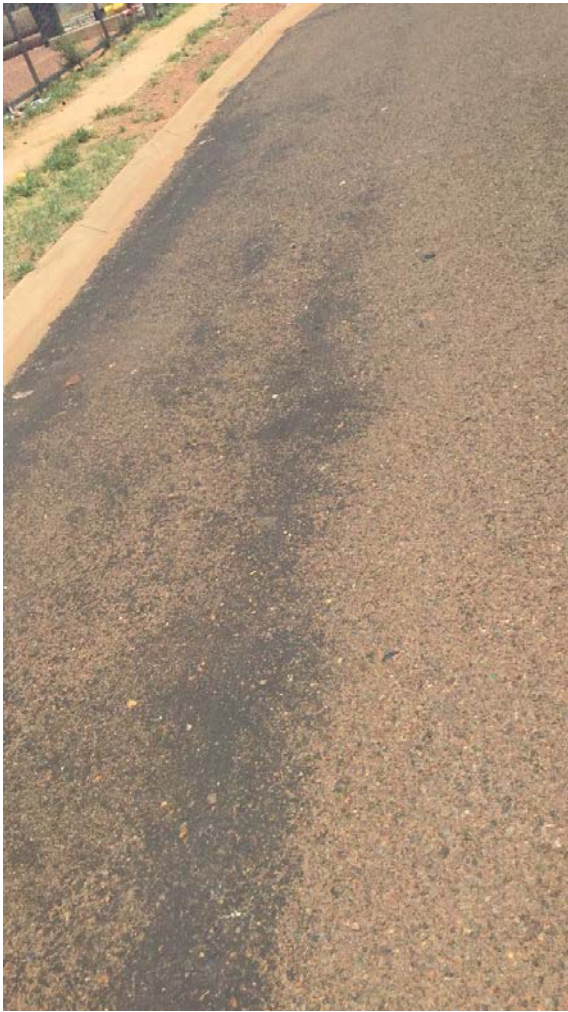
Figure 9 Road 215_1 with bitumen bleeding, condition: good
