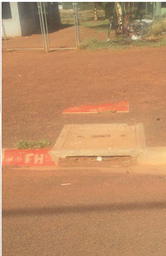
Figure 12 One bay side entry pit, condition: poor , blockage: 100%
