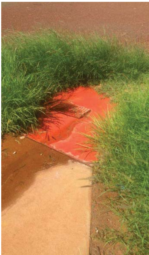
Figure 4 Fire hydrant, condition: poor
