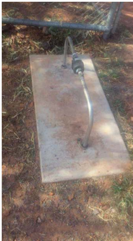
Figure 5 Water meter (lot), condition: poor
