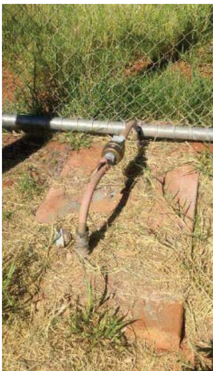
Figure 4 Water meter (lot), condition: good
