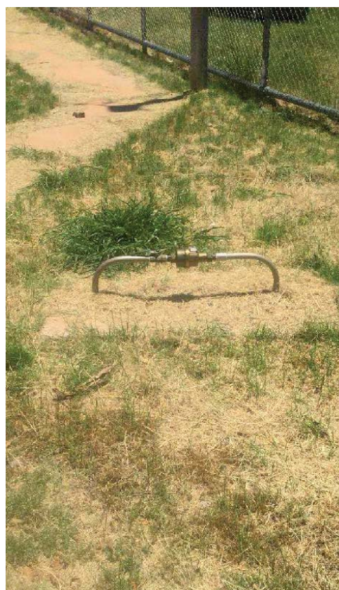
Figure 5 Water meter (lot), condition: good
