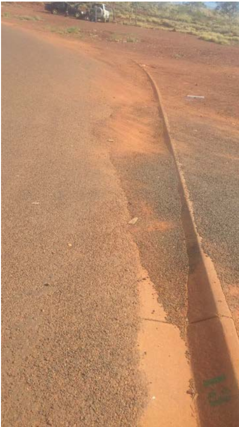
Figure 9 Road 238_4, condition: poor
