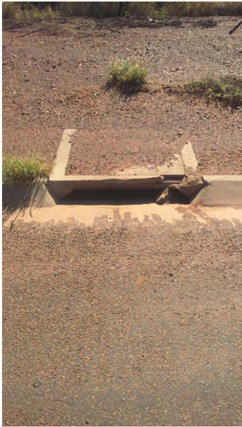
Figure 11 One bay side entry pit, condition: very poor
