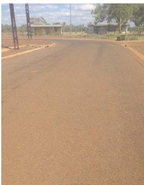
Figure 10 Wuppa Town Camp Internal Road, condition: good . Stone loss, bleeding defects
