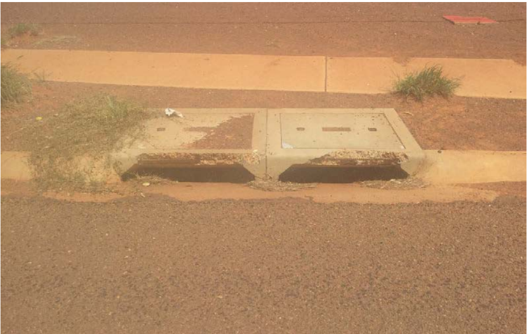
Figure 11 Two bay side entry pit, condition: poor
