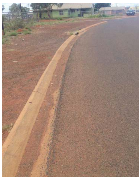
Figure 9 Wuppa Town Camp Internal Road, condition: good . Dirt in gutters
