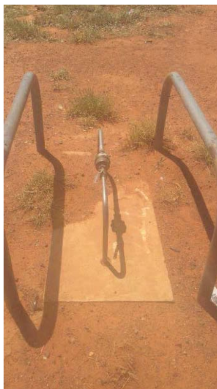
Figure 5 Water meter (lot), condition: good
