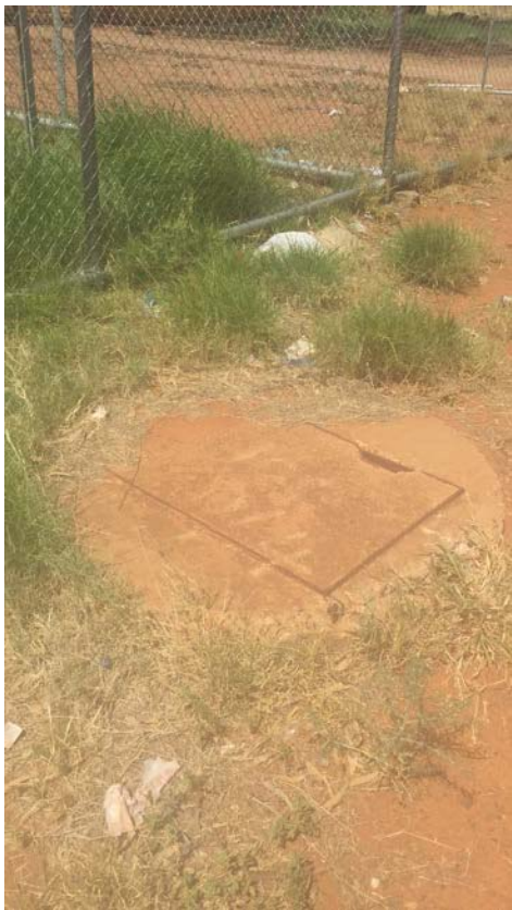
Figure 2 Sewer manhole, condition: poor
