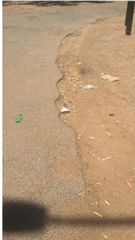
Figure 7 Edge breaks, condition: poor
