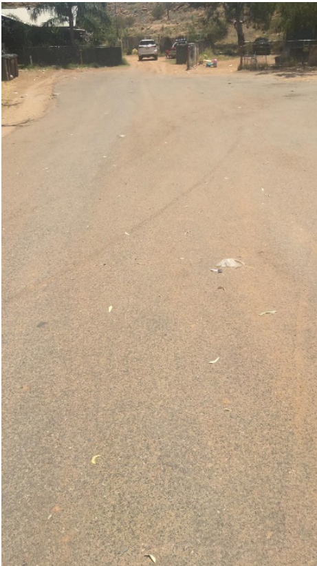
Figure 6 Pavement, condition: poor
