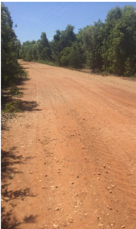
Figure 12 Pavement, condition: poor
