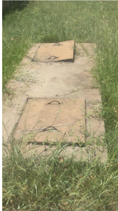
Figure 5 Sewer manhole, condition: very poor
