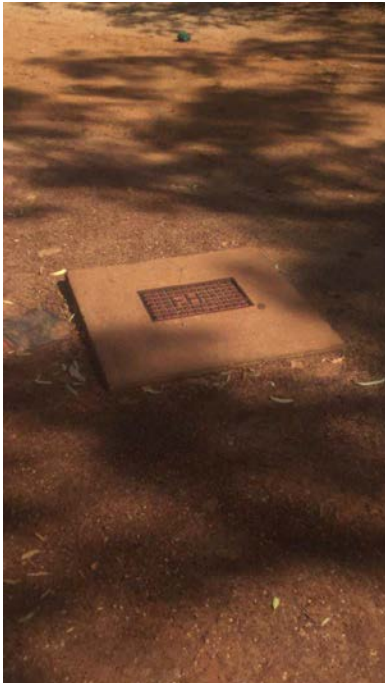
Figure 3 Fire hydrant, condition: good
