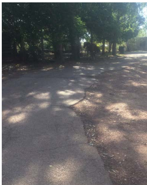
Figure 8 Road, condition: very poor
