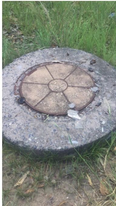
Figure 7 Sewer manhole, condition: poor
