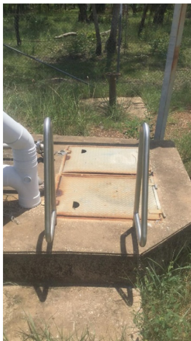
Figure 3 Sewer pump station (access chamber)
