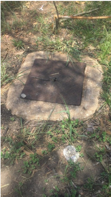
Figure 6 Sewer manhole, condition: very poor
