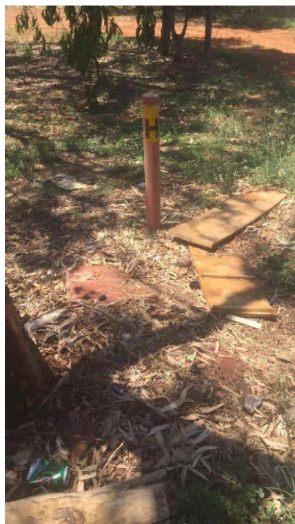
Figure 5 Fire hydrant, condition: poor
