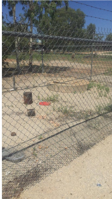
Figure 2 Sewage pump station, good condition
