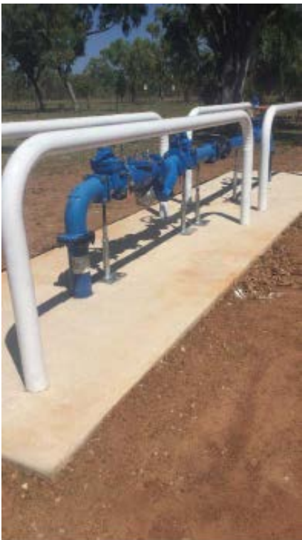
Figure 8 Water meter (bulk), condition: excellent
