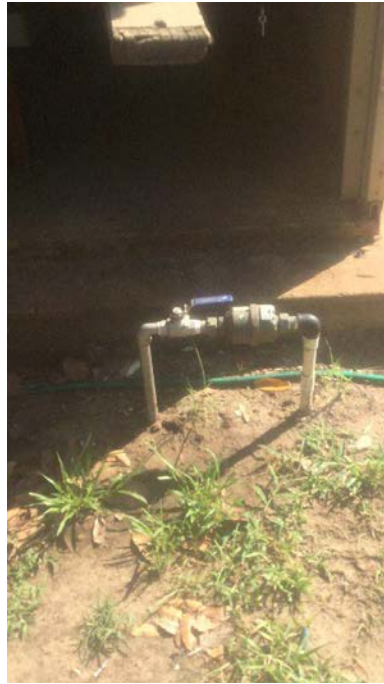
Figure 4 Residential lot water meter, condition: good
