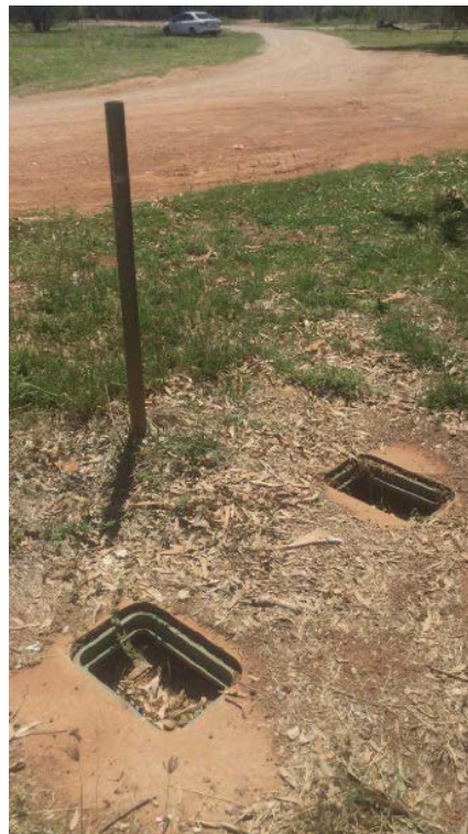
Figure 9 Water meter (lot), condition: very poor
