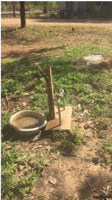
Figure 5 Tap, condition: good
