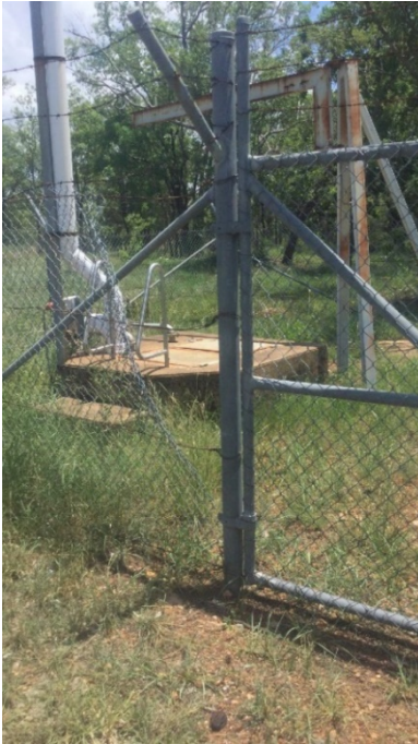
Figure 4 Sewer pump station (davit arm)
