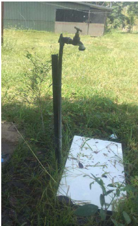
Figure 9 Tap, condition: very poor
