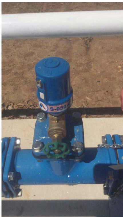
Figure 4 Air valve, condition: excellent
