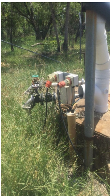
Figure 2 Sewer pump station (electrical)
