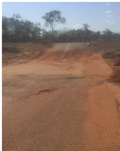
Figure 9 Garawa Two access road, condition: very poor
