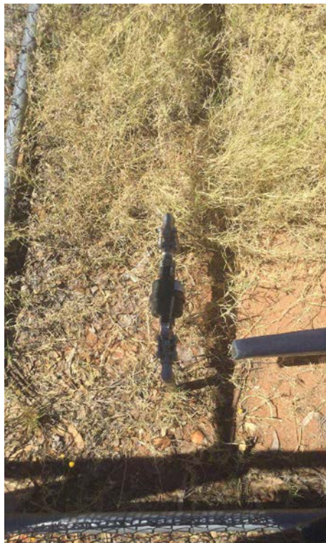
Figure 6 Residential lot water meter, condition: poor
