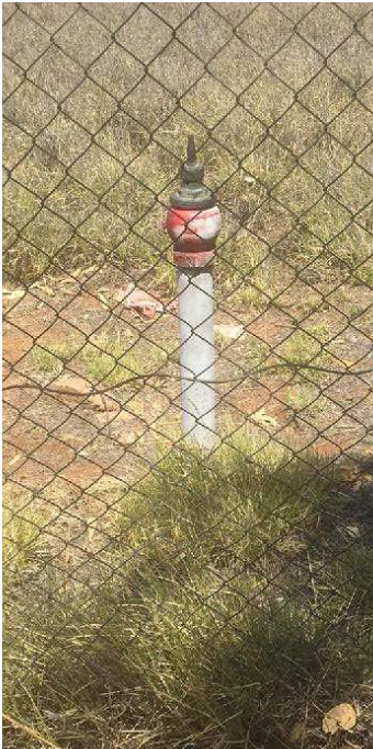
Figure 2 Fire hydrant, condition: poor
