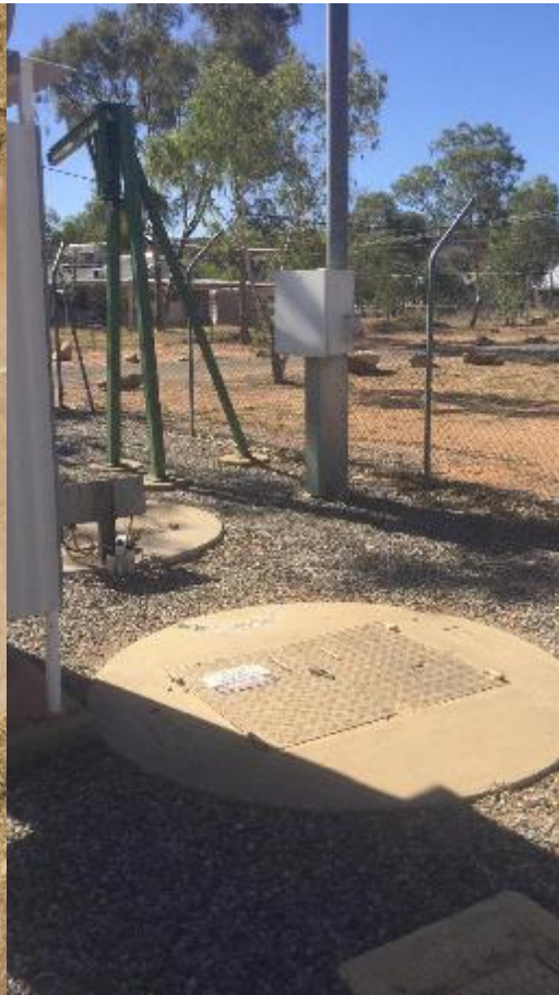
Figure 3 Sewage pumping station, condition: very good
