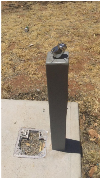
Figure 18 Bubbler, condition: very poor
