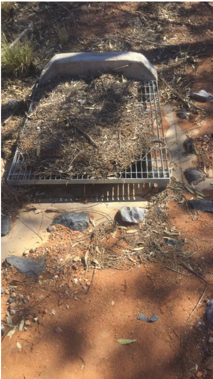
Figure 15 Letterbox pit, condition: good
