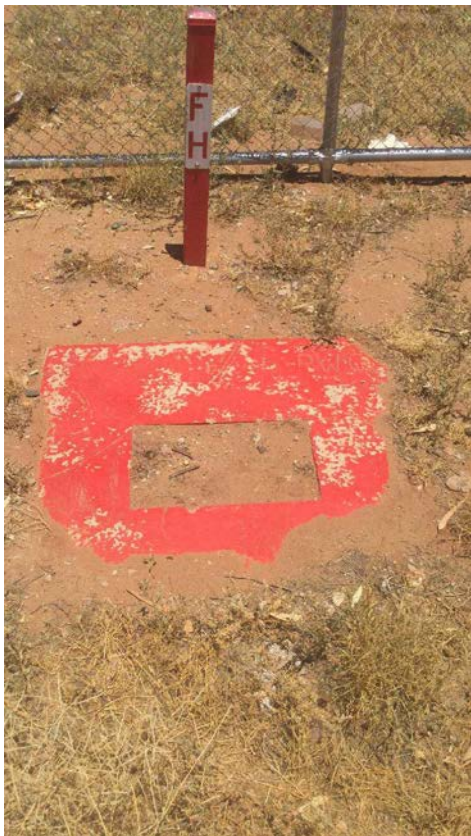
Figure 5 Fire hydrant, condition: poor
