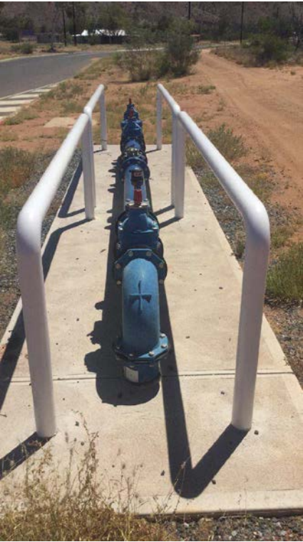
Figure 3 Water meter (bulk), condition: very good
