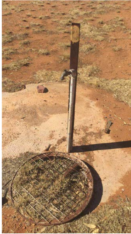
Figure 4 Tap, condition: very poor
