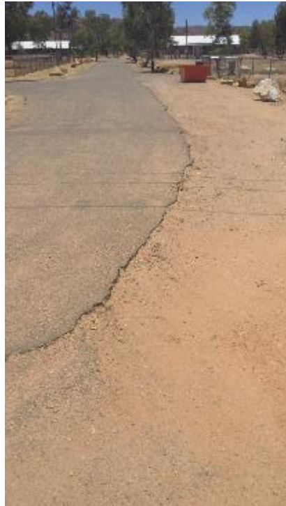
Figure 11 Edge breaks, condition: good
