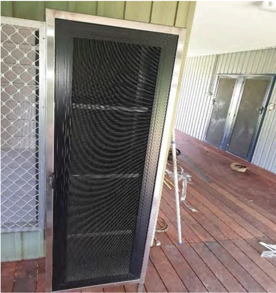
New decking in the living area and kitchen along with the pantry
