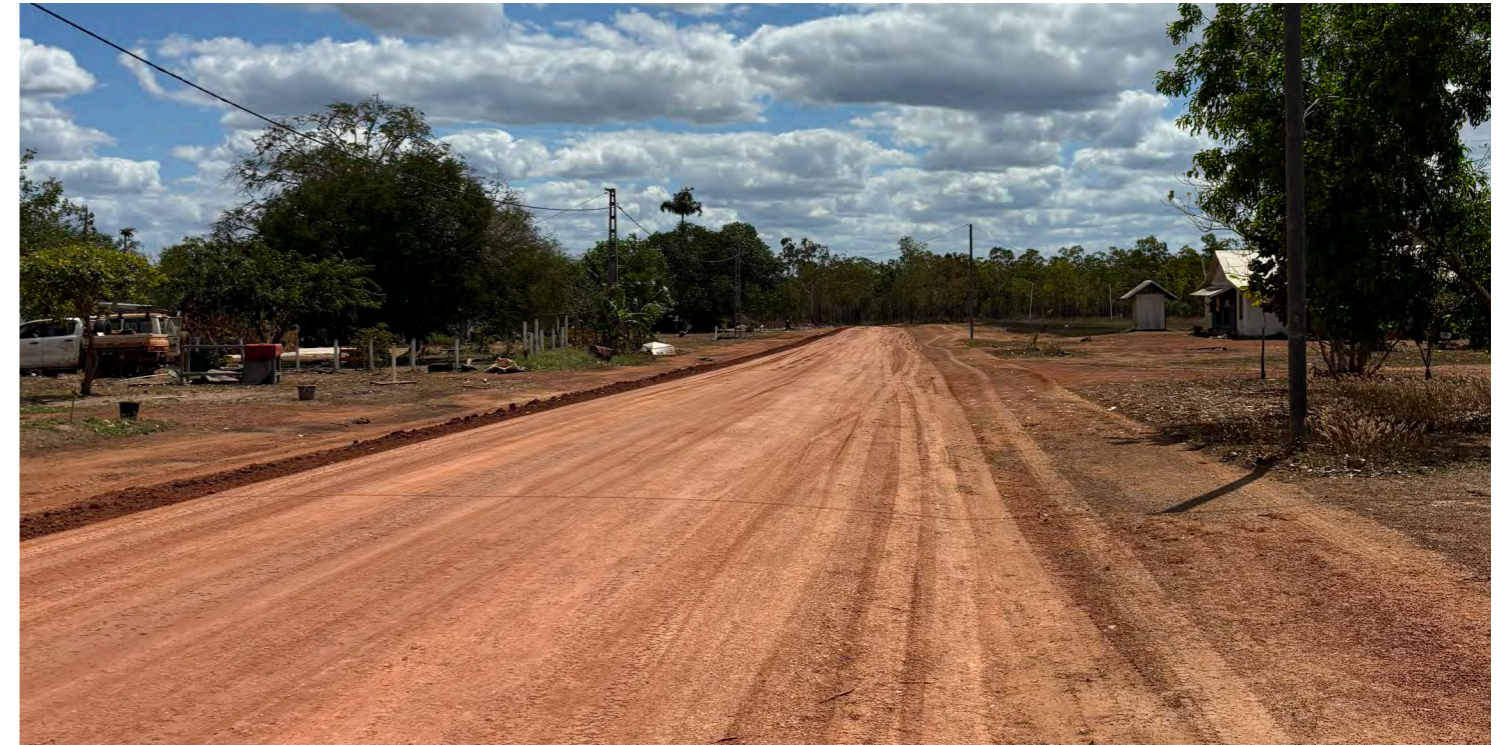
Photo of internal road works in progress, internal road running north/ south
