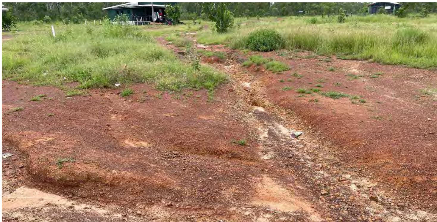
Before photo of stormwater damage to internal road, view towards east
