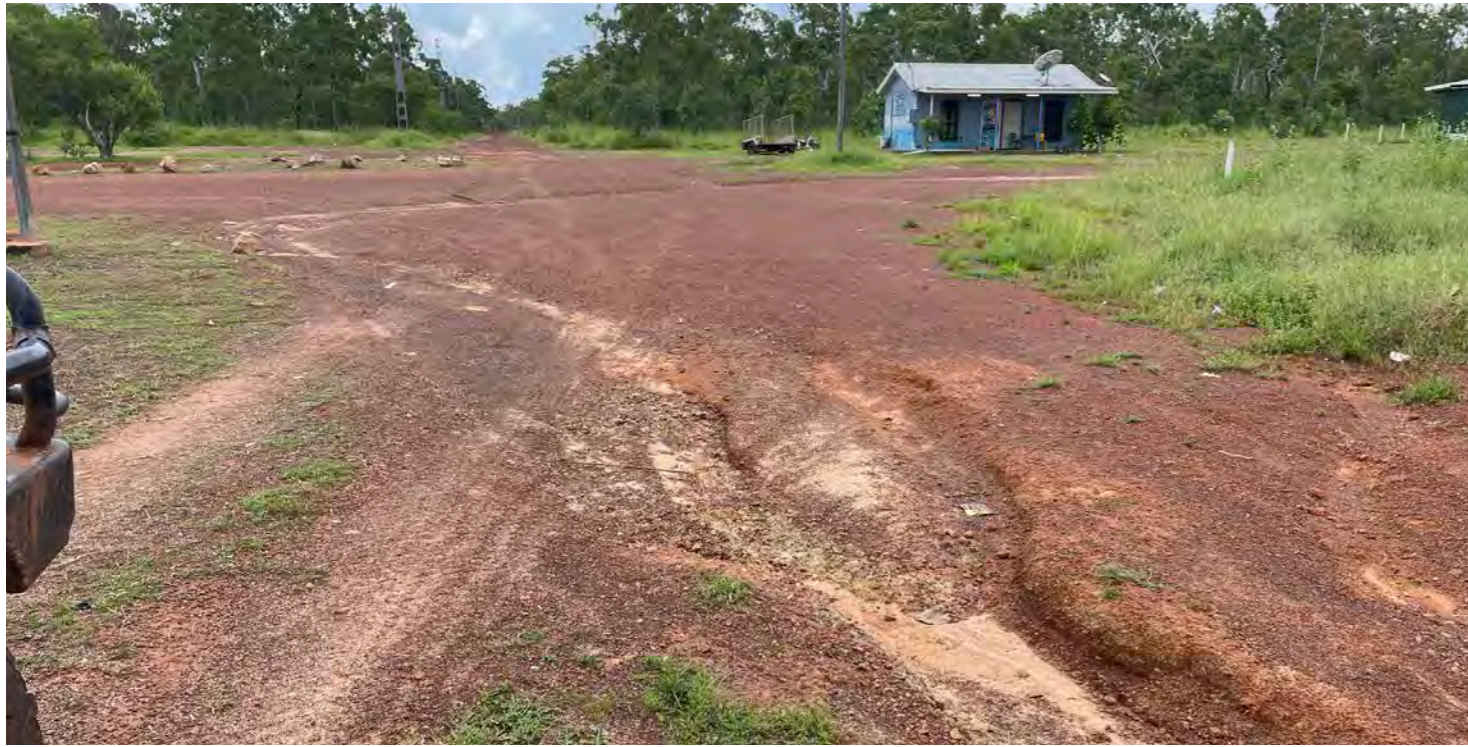
Before photo of stormwater damage to internal road, view towards north
